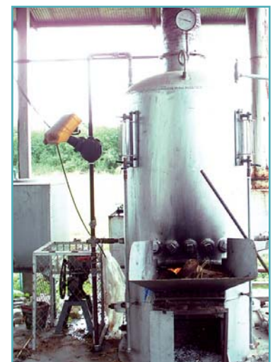
Figure 7. Steam generator for pasteurization
