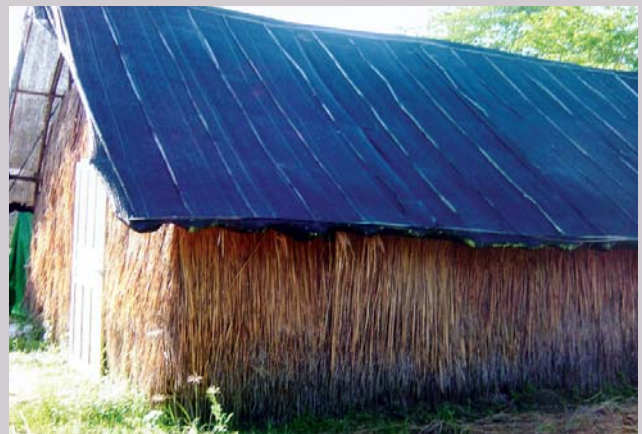
Figure 20. A mushroom growing house made up of dried grasses and bamboo wooden frame
